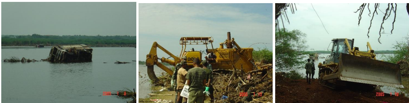
Komatsu 155, Komatsu 85 Crawler Tractors, PC 200 Crawler Excavators etc were used to remove the large vehicles partially submerged in the lagoon
